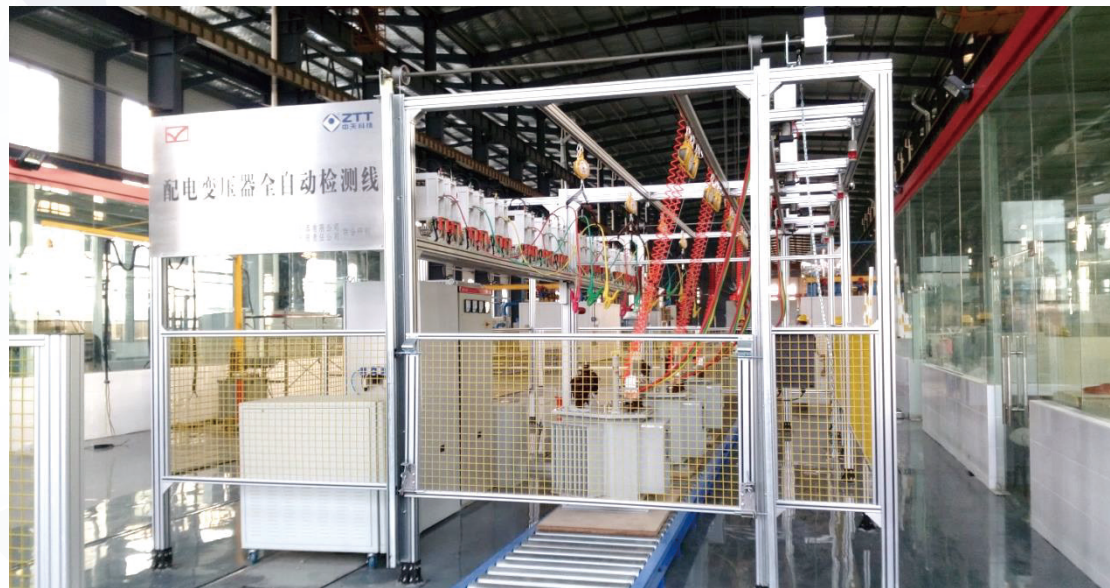
NKT Pipeline transformer test station
