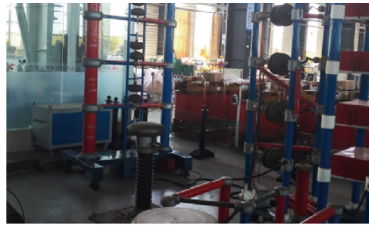
Impulse voltage generator
